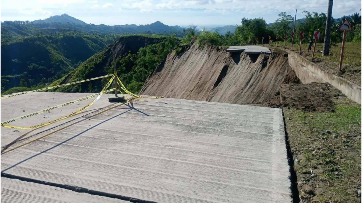
In photo: Road collapse in Barangay Tbolok, General Santos City (Photo Source: Barangay Tbolok / General Santos City via Facebook)
